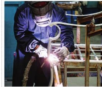
Components and parts are clamped in place in a welding fixture and welded using a full 360-degree circumference weld.
